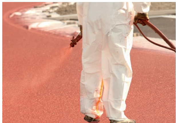
Regupol® topseal UV is applied as a spray on the top of the sports flooring.
